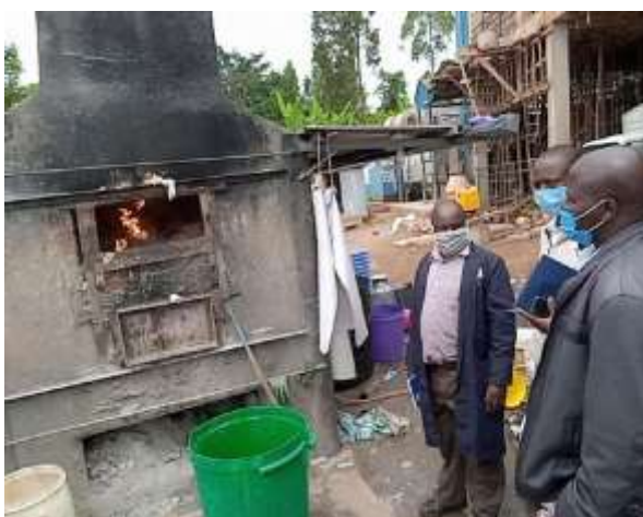
Incinerator at Wakulima dairy
