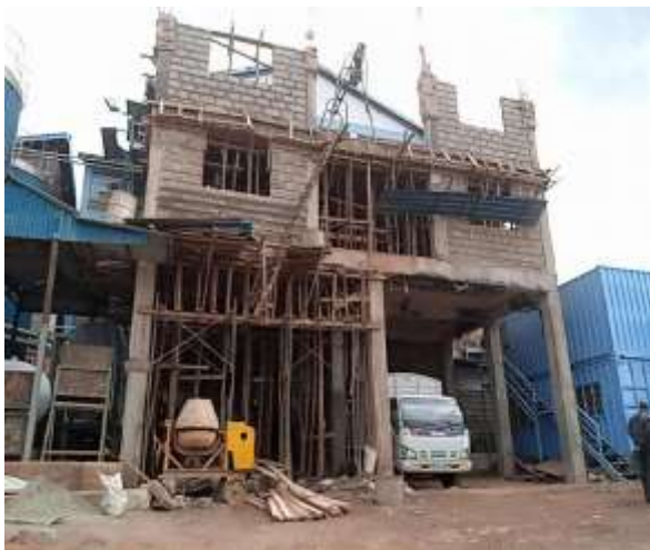
The proposed Tetra Pack Fino Extension Unit already under construction at Wakulima dairy
