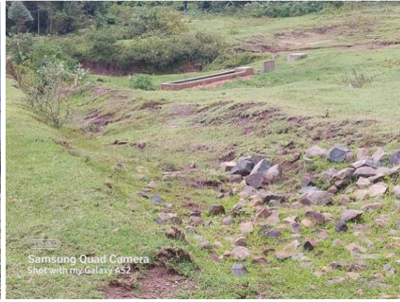
Plate 4: Gulley developing at the spillway
