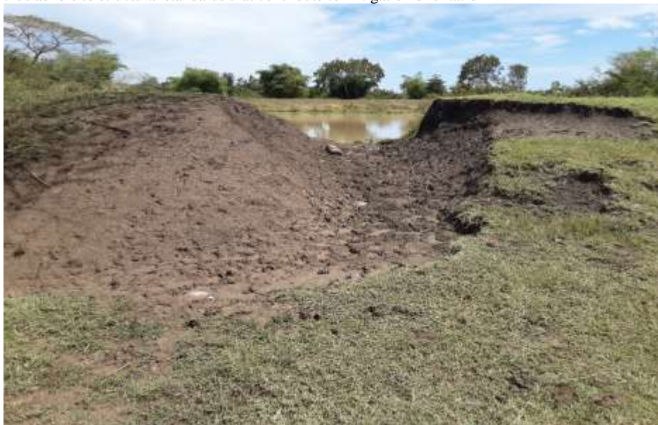
Plate 3: Breached embankment of the existing water pan to be rehabilitated
