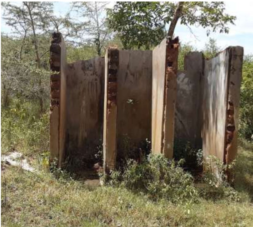
Plate 4: Dilapidated toilets at the current site
