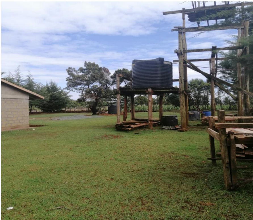
Figure 3.7: Water storage tanks at Timor Cooperative Society
