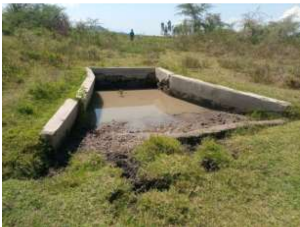
Dilapidated Water Point (Require CWP and LWT)
