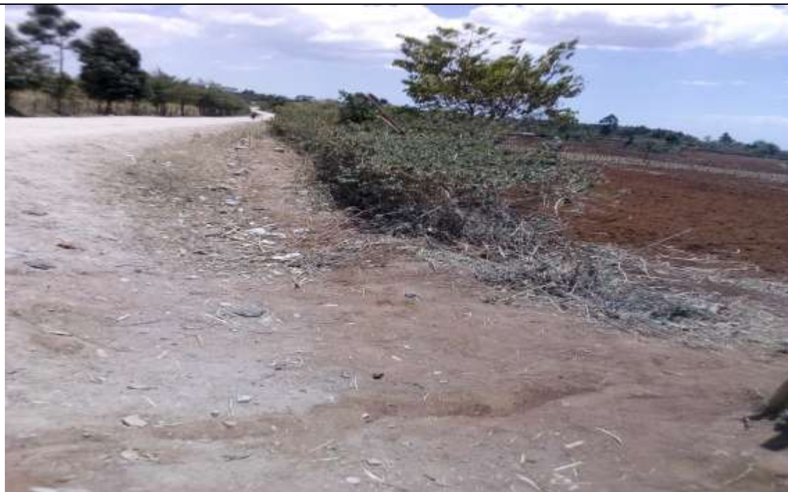
Figure 4: Photo of Marram Road Contributing Run-off Water Discharge into Chepchirik Water-pan
