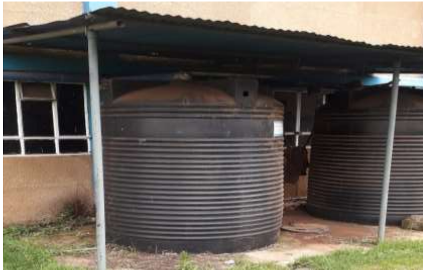
Plate 1: storage tank for roof water harvesting
